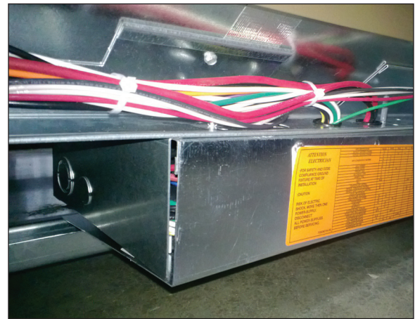
Fig. 15 Junction box beneath case
